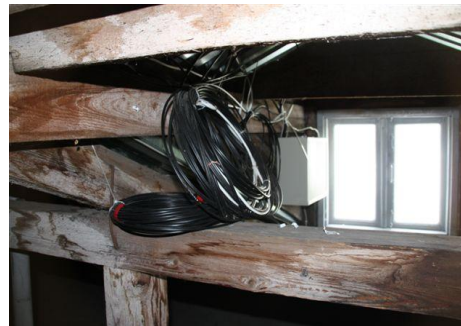
5.) wiring on roof
