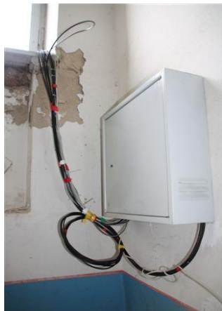
11.) wiring to control box
