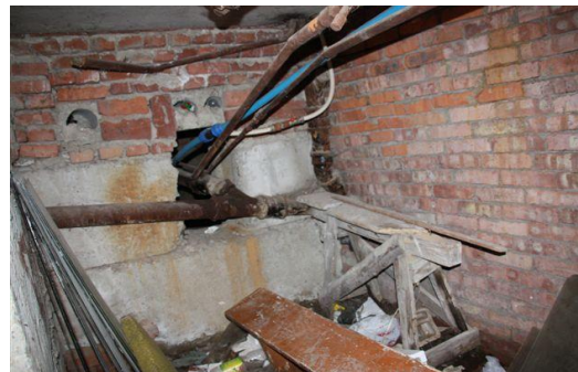
5.) waste and poor condition in underground floor
