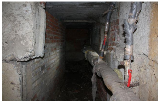
4.) poor piping insulation in underground floor
