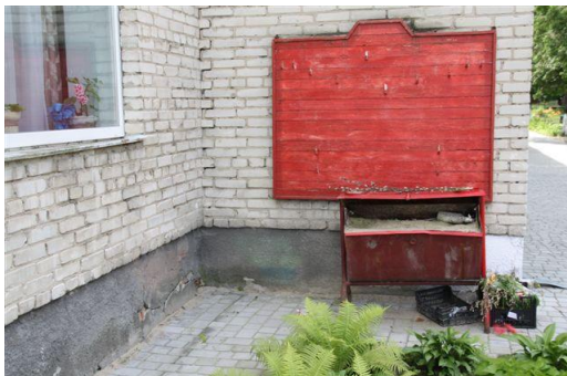
4.) no fire fighting equipment
