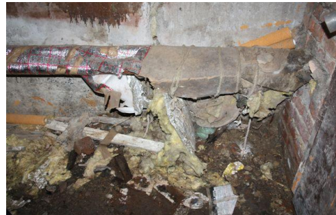
8.) waste in underground floor
