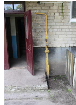
14.) external gas piping
