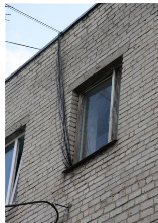
12.) wiring to control box (street view)
