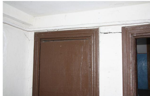
5.) cracks in walls inside
